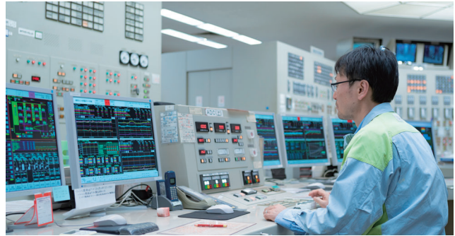
Central Control Room
